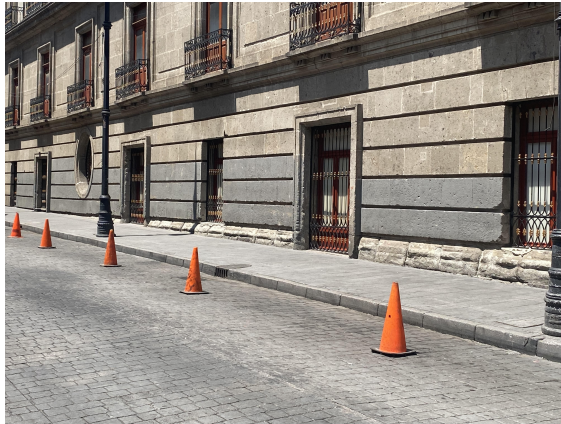
(c) Building whose foundation is exposed on one side as pavement sinks unevenly around it, downtown Mexico City
