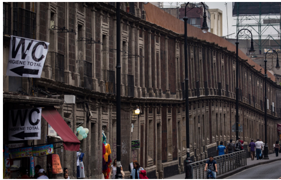
(a) Building distorted by uneven sinking in one side in Texcoco, downtown Mexico City
