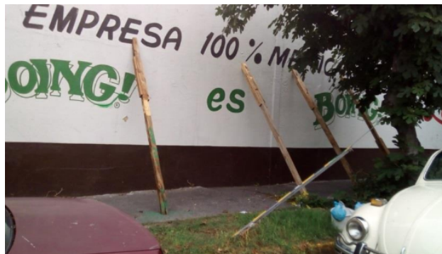
(e) Wall tilting into sidewalk, Venustiano Carranza
